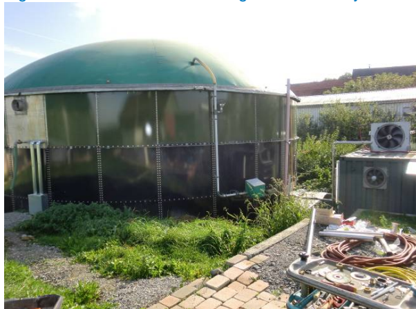
Figure 3-7: Farm-based bio-digester. Germany
