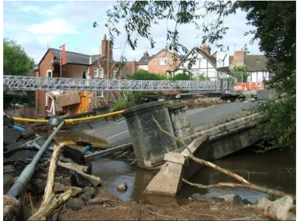
Flood damage on Burway Bridge, Ludlow June 2007 By DI Wyman, CC BY-SA 2.0, https://commons.wikimedia.org/w/index.php?curid=13997411
